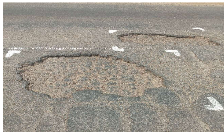
Figure 4. Delaminated road surface
