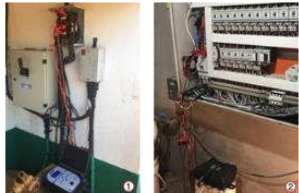
Figure 19. Electrical energy analyzer properly installed in poultry houses (1) A1 and (2) A2 respectively
