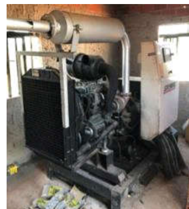
Figure 15. Stamac generator system
