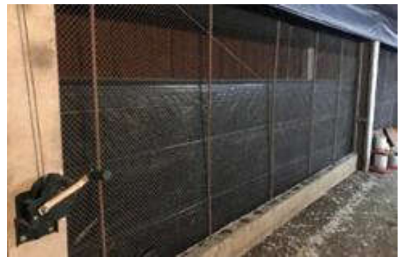
Figure 13. Cooling system - Pad cooling with air control performed with manual activation of the curtains
