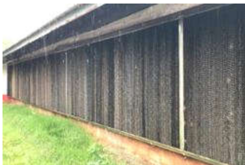
Figure 12. Cooling system - Pad cooling - Face 3
