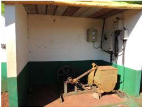
Figure 11. Nova brand three-phase New Bei line synchronous generator system
