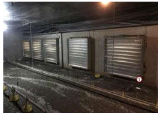
Figure 14. Ventilation system - Exhaust fans. Face 3 - Internal view. (1) Exhaust fans in operation, but not active
