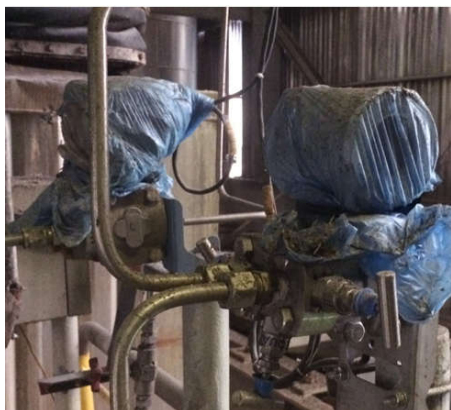
Figure 14. Differential Pressure Transmitter Installed
