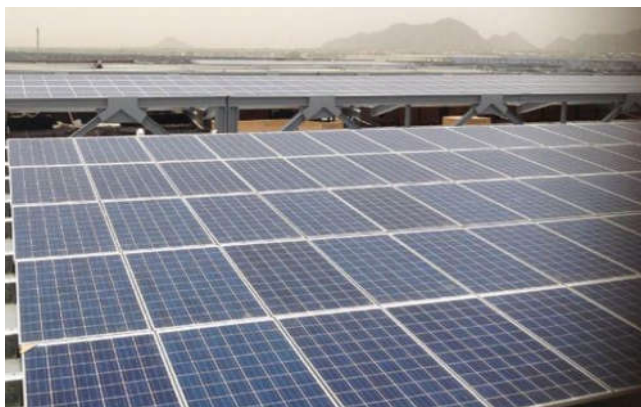
Figure-3.6. Mounting Structure of SPV
